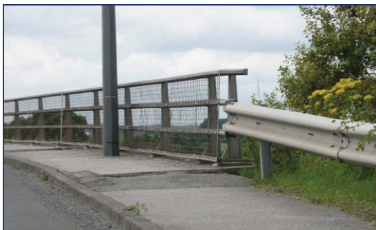
② Evidence of footway subsidence on embankment
