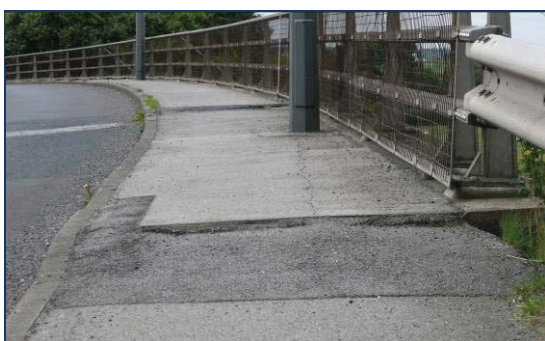
③ Uneven footway surface at subsidence location
